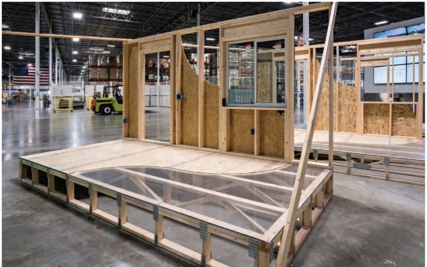
Katerra wants to cut costs by reducing options and making more of its own materials—even engineered lumber
